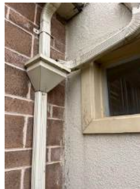
Crack along the corner.
